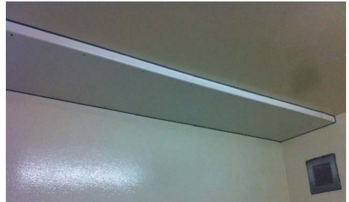
Above, NOMS ceiling mounted panel in a cell at HMP Blundeston
