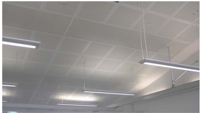
Above Trident ceiling grid panels at Kemball School, Stoke
