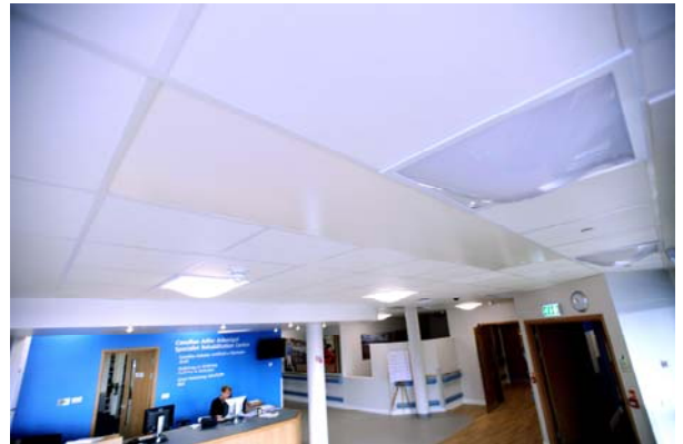
Above , Trident ceiling panels at Morrilton Hospital, Swansea
